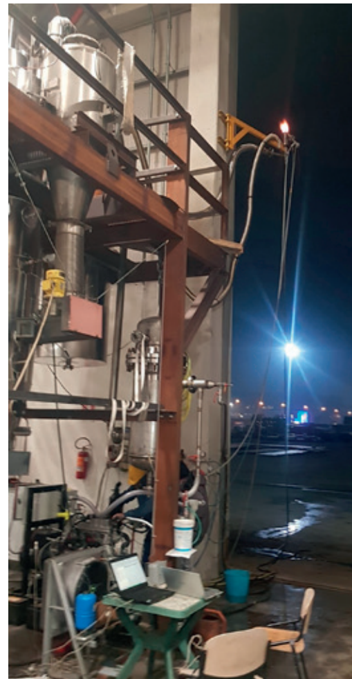
The fluidised bed gasifier that is producing syngas via nuts shells
