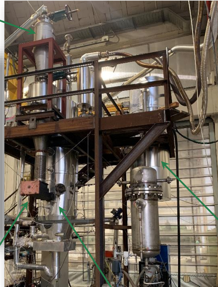
Dual bubbling fluidized bed gasifier
